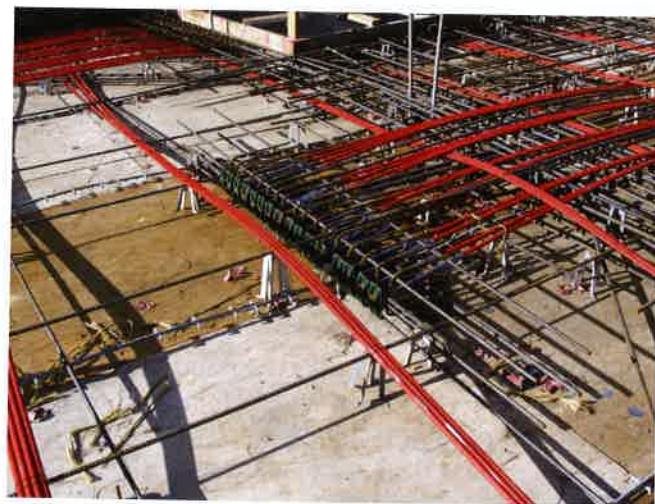
FIGURE 8.6-7 Unfavorable Termination of Tendons All at the Same Location. Stagger dead ends and provide bars to spread tendon force to front of anchors. (P726)
