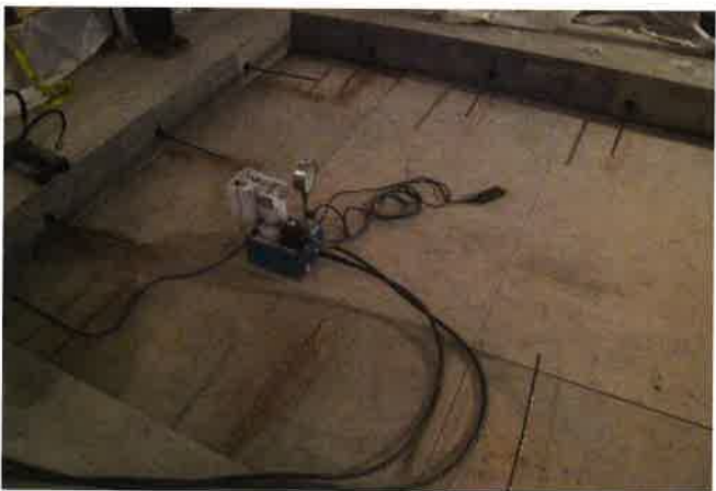
FIGURE 9.4-6 View of Tendons Re-anchored at the Edges of a Large Opening Made in an Unbonded Floor System (San Francisco; P735)
