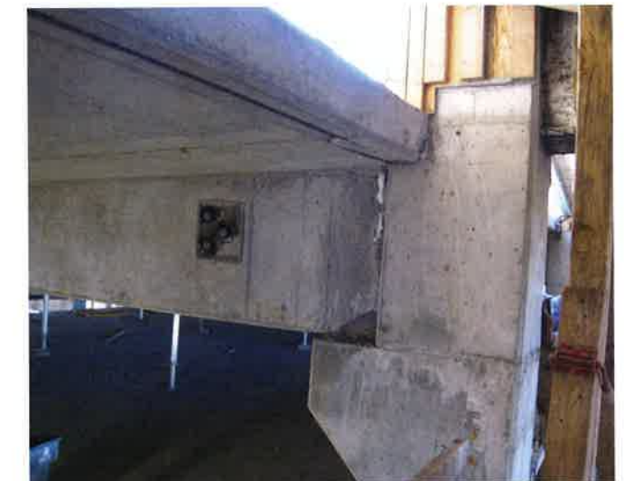
FIGURE 8.6-2 Tendons Cross Over and are Stressed at the Sides of the Beam, Where Tendons Can Not Extend Through The Column (California; P730)
