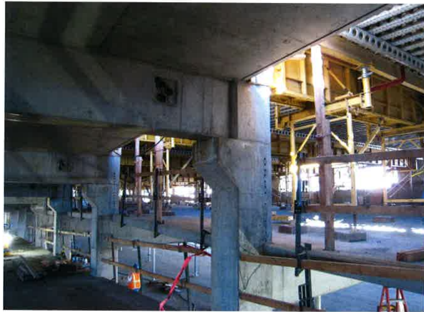
FIGURE 7.SI.1 Beam and Slab Construction; Beam Released from Column; Tendons crossed and stressed on stem sides (California; Courtesy DES and ADAPT; P731)
