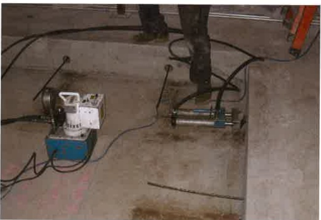
FIGURE 9.4-5 Stressing at Edge of Large Opening Made in an Unbonded Floor System (San Francisco; P734)
