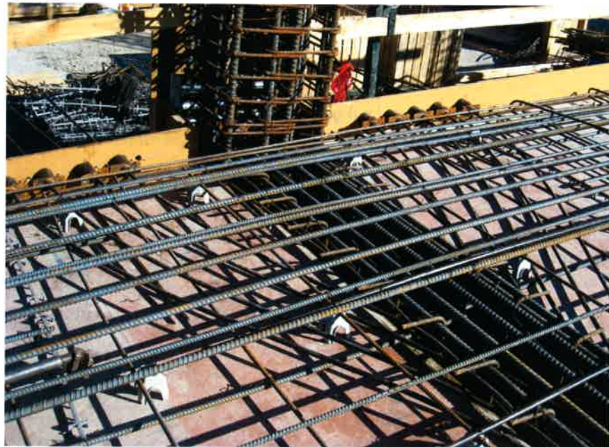
FIGURE 7.SI.2 Beam and Slab Construction; Monolithic Beam-Column Connection; A number of tendons are crossed over within the beam stem and raised to anchor at slab edge (California; Courtesy DES and ADAPT; P732)
